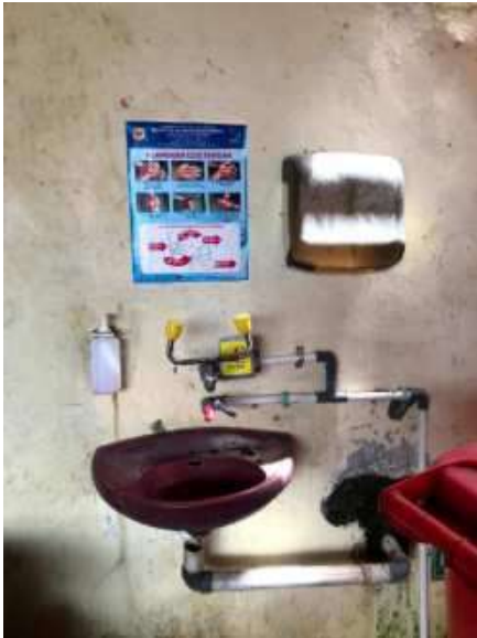
Gambar 5. Kran Air TPS
