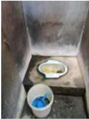
Jenis jamban non septic tank
